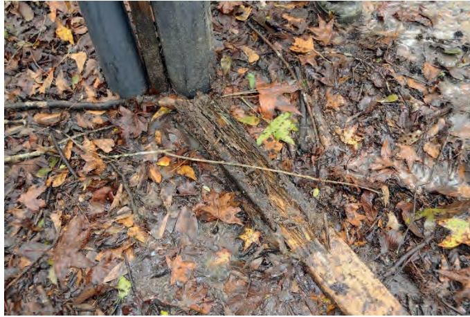
Figure 5. This feeder stake was consumed by Formosan termites to the point where it fell over.
