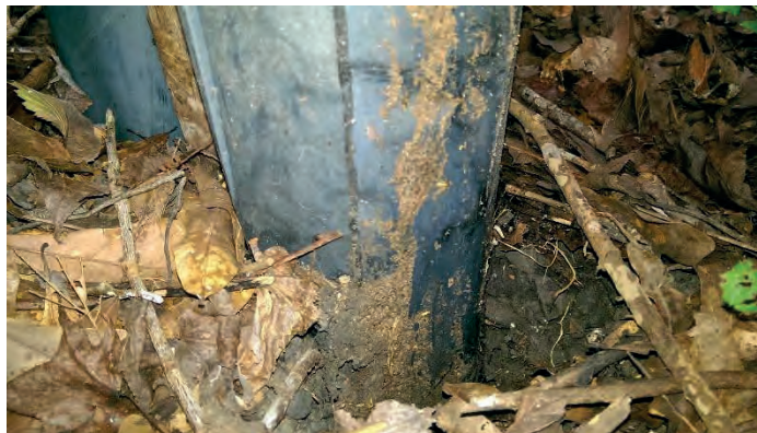
Figure 4. Signs of Formosan termite feeding pressure on the butyl copper foil/poly tape.
