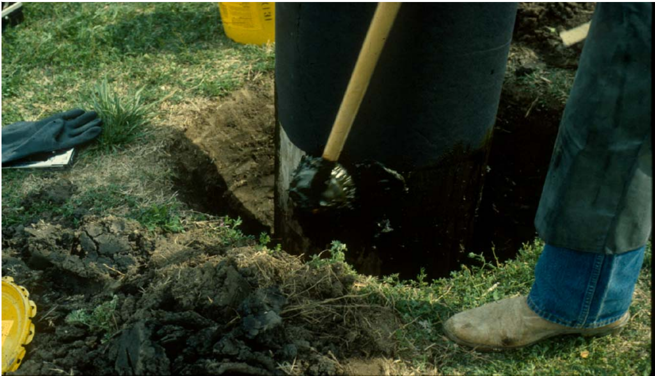
Figure IV-2. Example of an external paste being brushed onto the below ground surface of an in-service utility pole.
